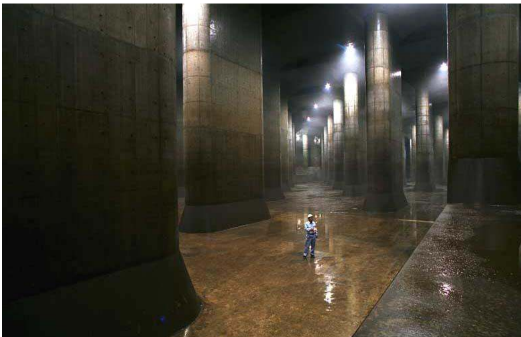
Figure 3: Azami hydrosphere processing plant during testing (G-Cans)
